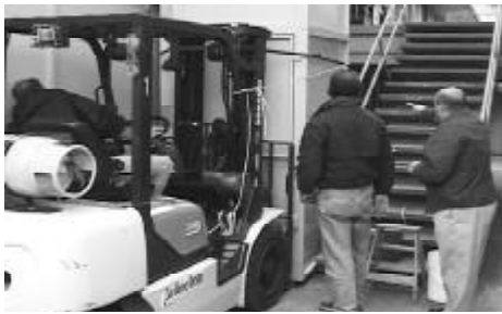
Tony with ADA certified contractor, Jana Construction during the harrowing installation process
